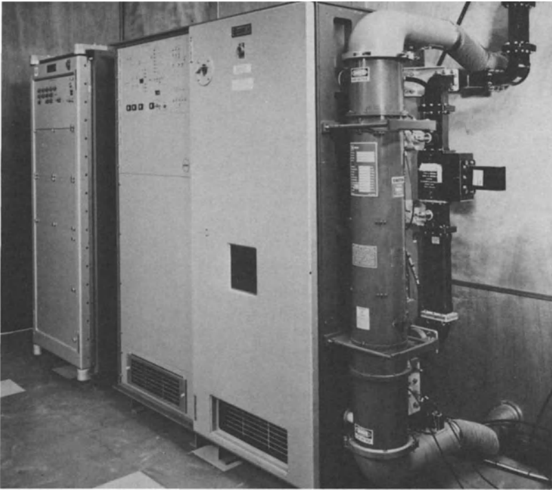
Figure 4.3 Transmitter–receiver cabinets and travelling wave tube of the Watchman S-band surveillance radar. Note the air-cooling ducts for the TWT, and the waveguide run to the antenna. The TWT power output is about 60 kW peak, 1.2 kW mean. A number of advanced features are incorporated, including pulse compression (photo courtesy of Plessey Radar Ltd)
