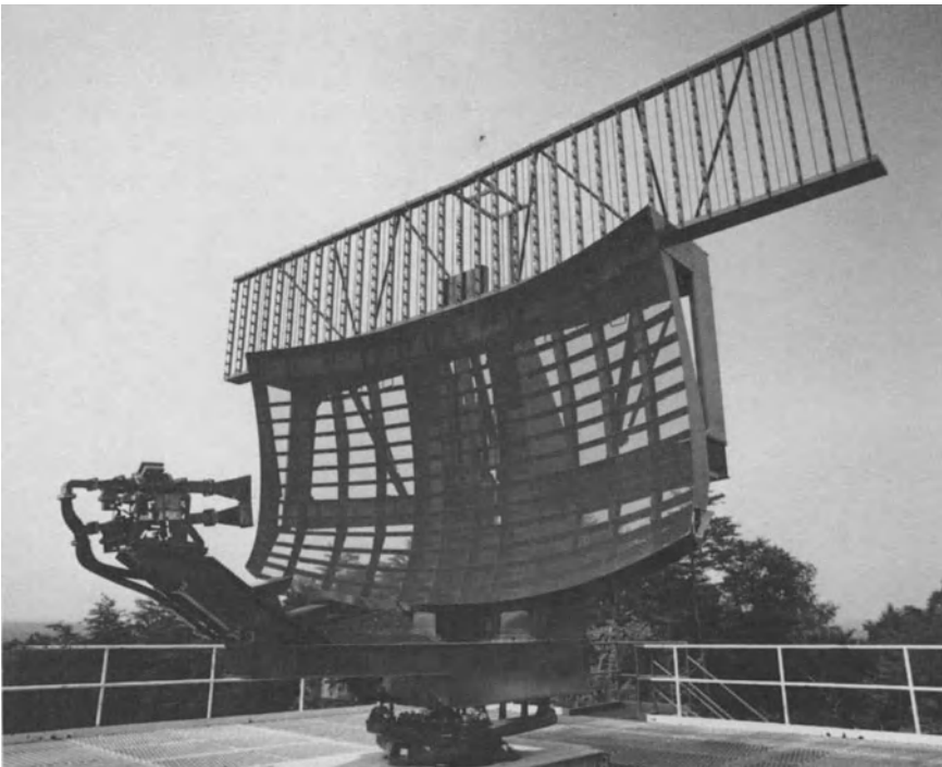
Figure 7.6 ASR-9 antenna, with co-mounted SSR (photo courtesy of Westinghouse Electric Corporation)
